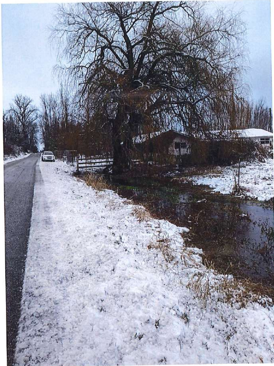
Photo 3: The ditch appears to bottleneck as it approaches the culvert crossing. Ditch continues to have a fair amount of vegetation.
