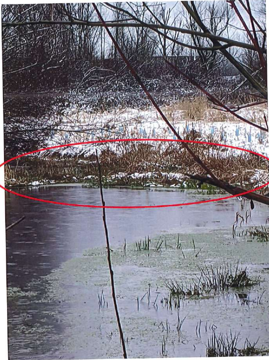
Photo 6: There appears to be a blockage in the channel just after the culvert crossing.
