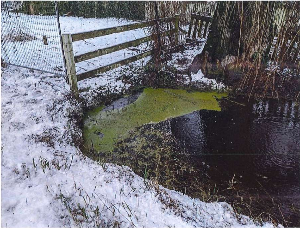
Photo 4: Upstream of the culvert inlet. Flow depth is roughly 5.5-ft to 6.5-ft and the top width is roughly 13-ft to 15-ft in this area. Culvert is fully submerged and could not be surveyed at this time.
