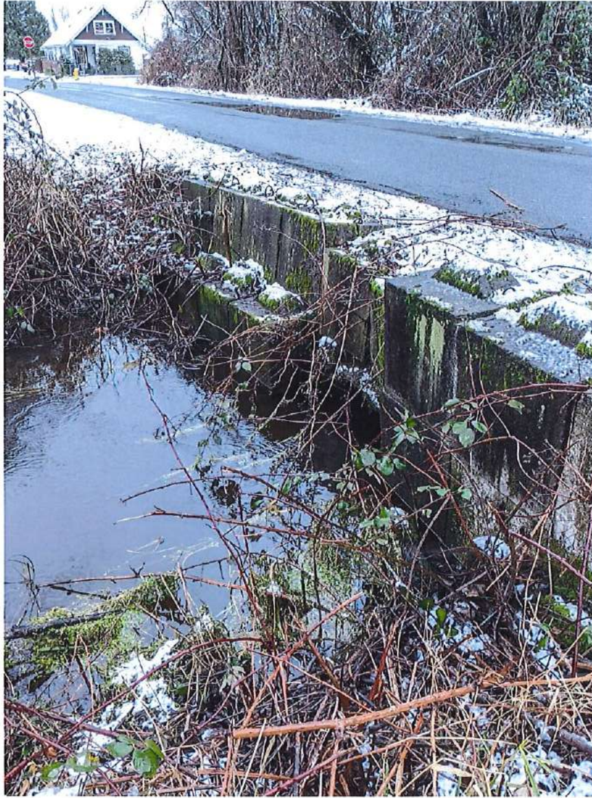
Photo 8: There are large culverts in the creek downstream of the project site. They were estimated visually to be roughly 4-ft in diameter. Conditions made it difficult to access the culverts safely for an accurate measurement.
