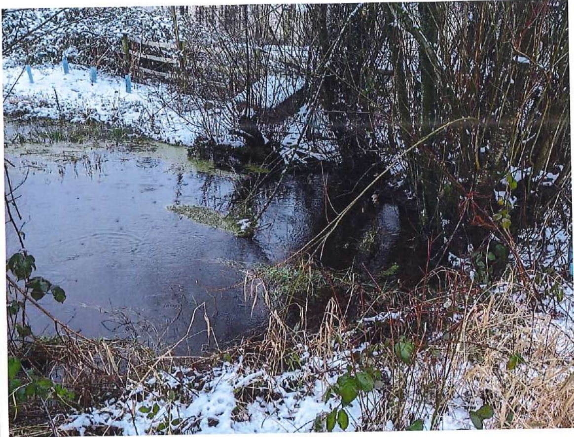
Photo 5: Ditch after the culvert crossing widens. Culvert is submerged and could not be surveyed at this time. Submergence is likely caused by an offsite downstream flow obstruction.
