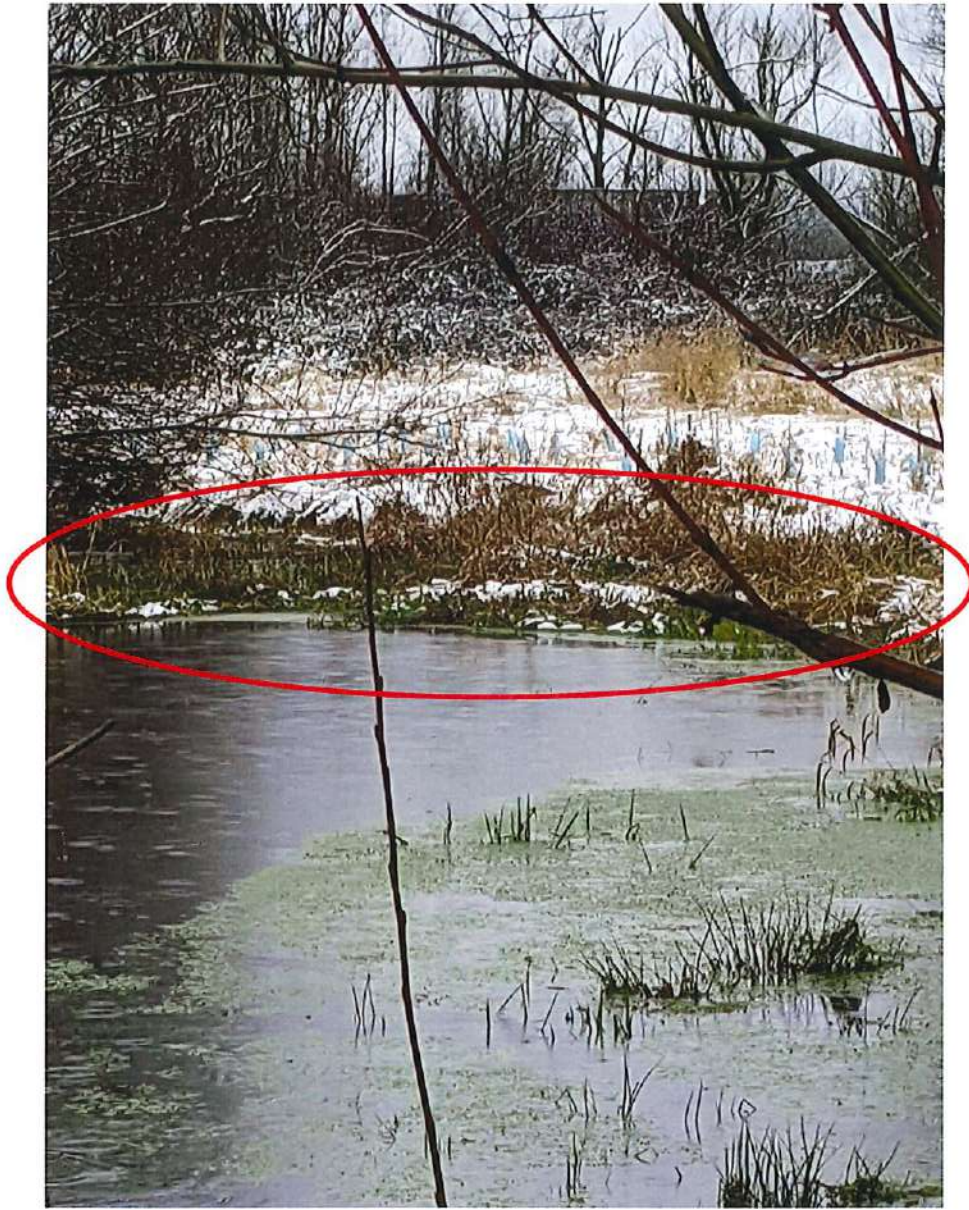
Photo 6: There appears to be a potential blockage in the channel just after the culvert crossing. Conditions made it difficult to access the area safely for assessment.
